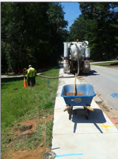
City of Stockbridge Oakland Boulevard Storm, Sewer, and Drainage Improvements, Stockbridge, Georgia
